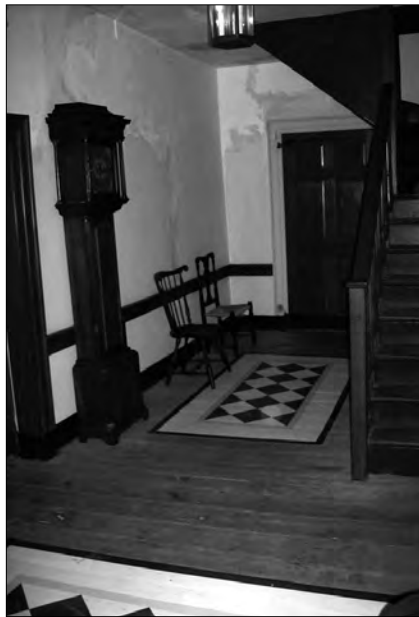
A view of the passage showing the removal of the door and plaster restoration.
